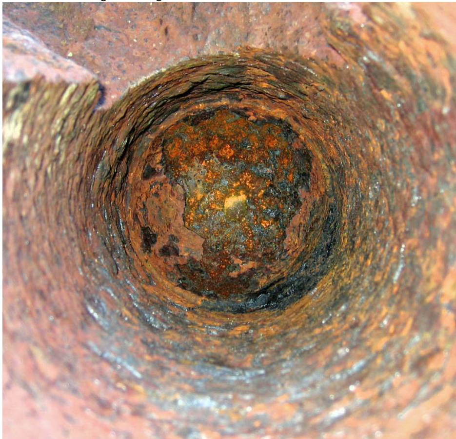
Image showing bore and outer face of ball after water blasting and scraping loose rust from bore. Ball was later removed.
