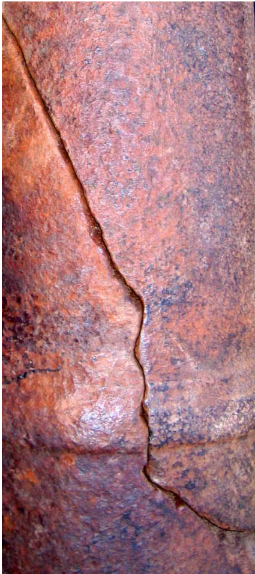
After water blasting and wire brushing - area showing the mating of the two broken barrel parts. Traces of the black surface coating applied c1955 still showing.
