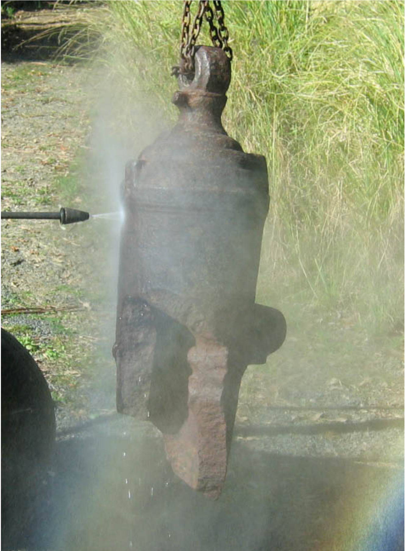
Water blasting using a turbo nozzle, this process was repeated several times to dislodge surface rust and growths.
